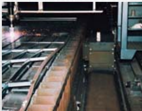
Belt duct and suction area
